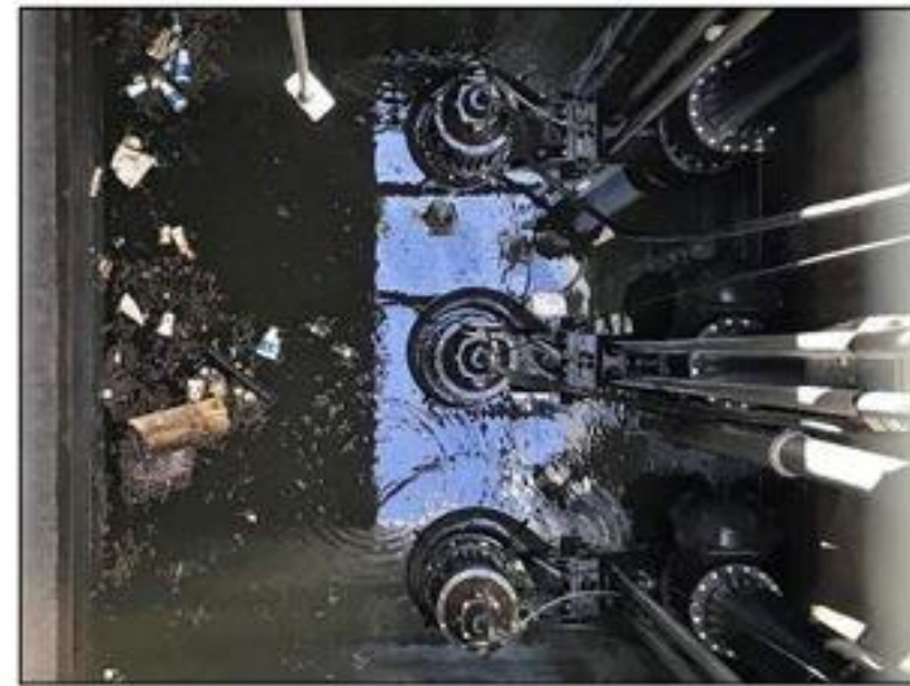
Photo 58 – Crossroads Submersible Pumps
