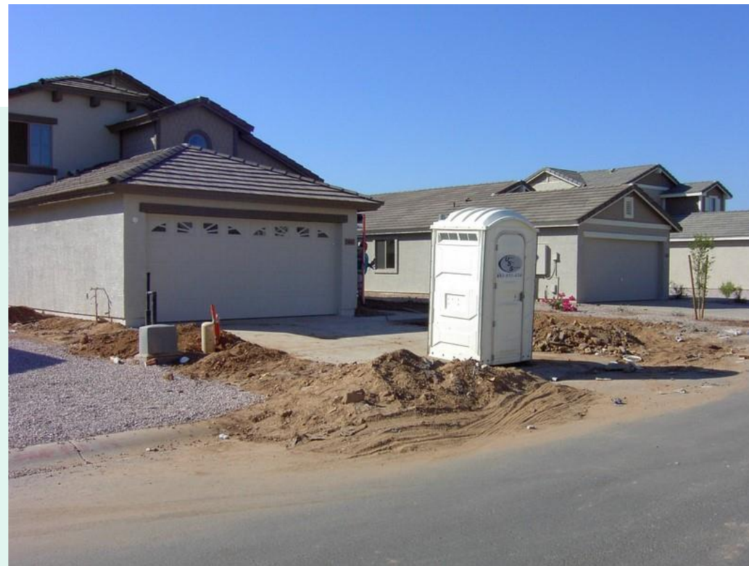
Construction sediment and debris not properly contained
