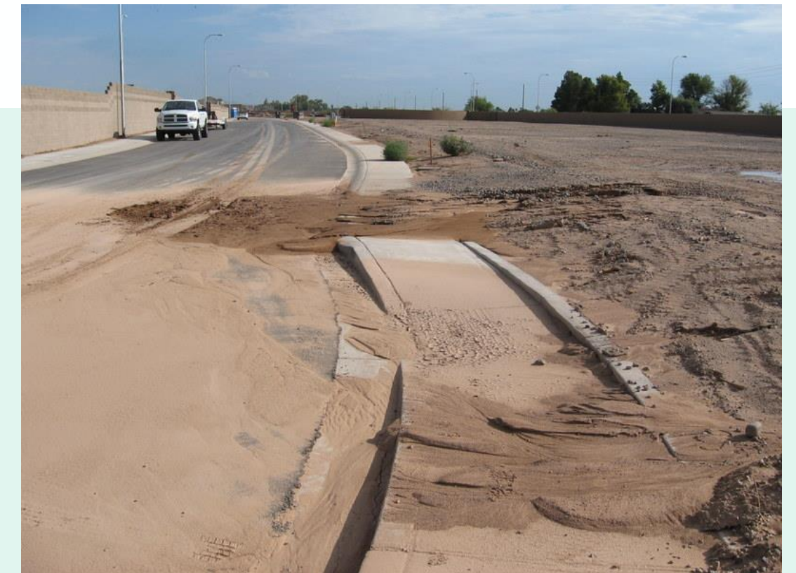
No barrier to prevent sediment runoff into streets
