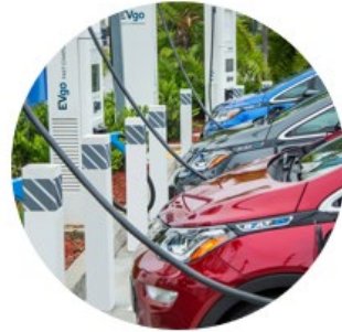
Electric vehicle charging
