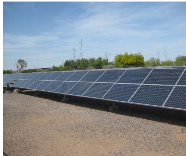
Gilbert APS Solar Power Plant
