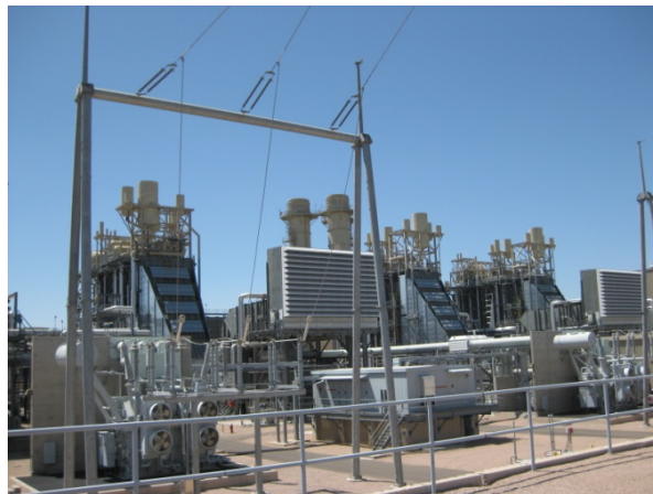
Santan Generating Plant
