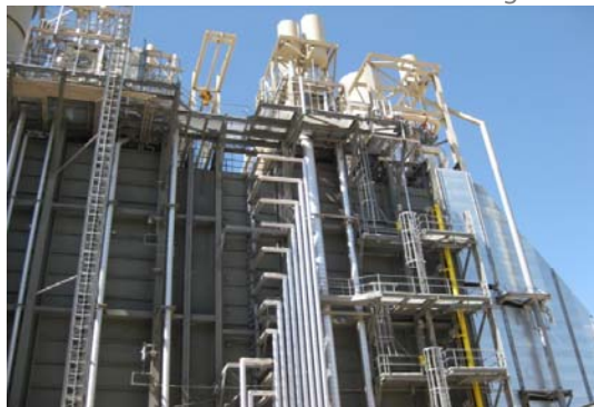
SRP Santan Generating Plant
