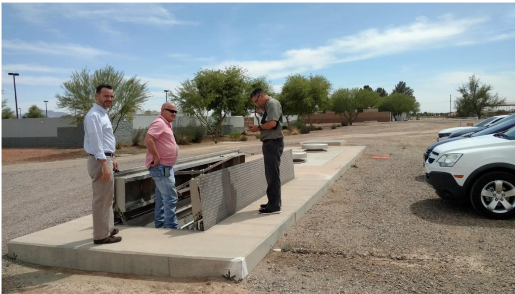
Below Grade Vault Entry Hatch and Ventilation
