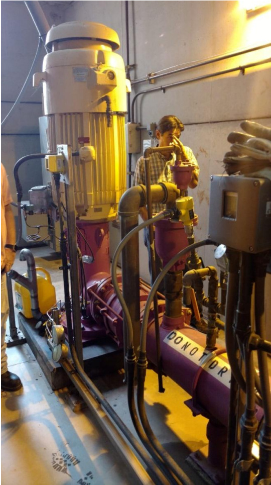
Well Pump and Recharge/Purge Line (flow in both directions)
