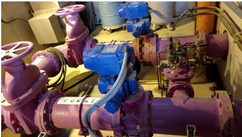
Reclaimed Water Recharge (top) and Purge (bottom) Lines
