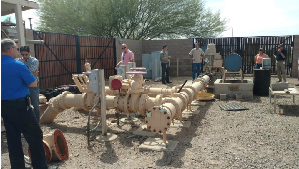
Reclaimed Water Recharge and Purge Lines
