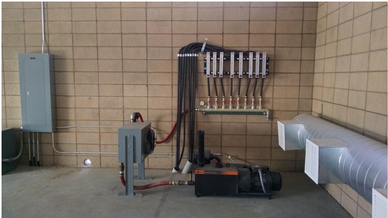
Example of Lake Aeration Mechanical System Installation
