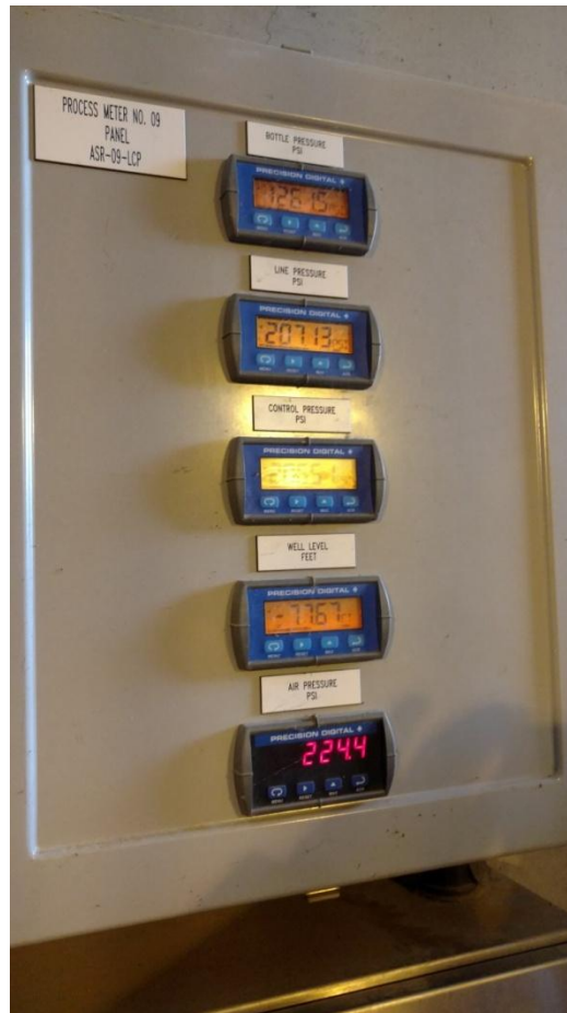
ASR Well Monitoring and Control Panel
