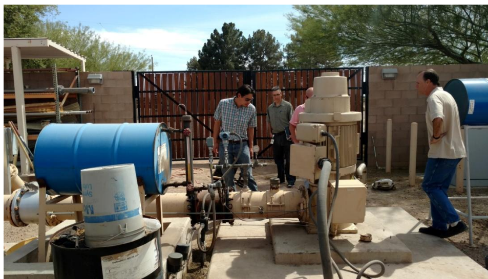
Well Pump and Recharge/Purge Line (flow in both directions)
