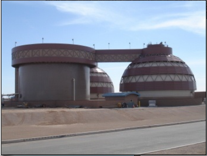
Greenfield Wastewater Treatment Plant
